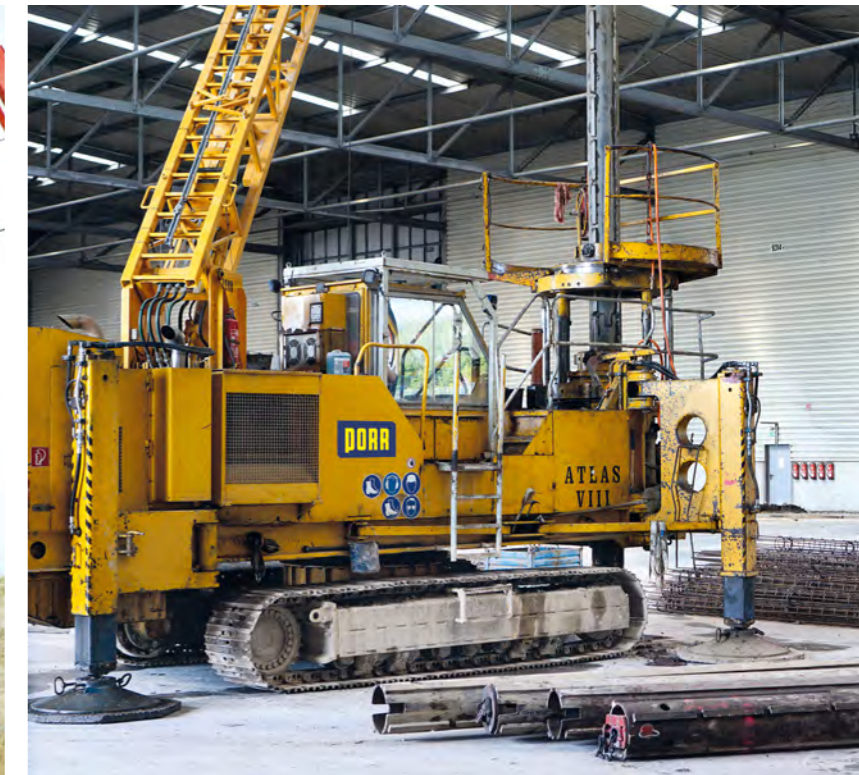
Due to the limited working height, the drill pipes are inserted in several shots and the reinforcement cages are rammed several times.
