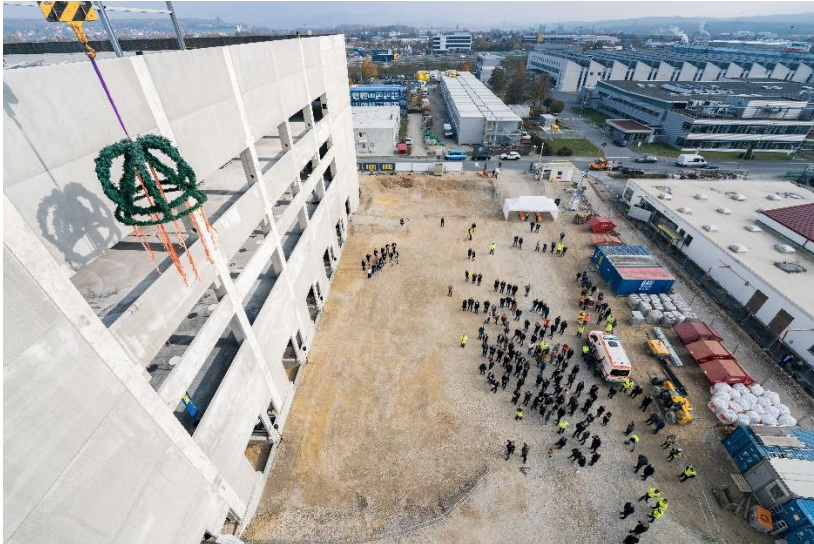
Caption: Topping-out ceremony of the High Energy Photonics (HEP) Center for Siemens Healthineers in Forchheim, Germany (Copyright: © Siemens Healthineers)
